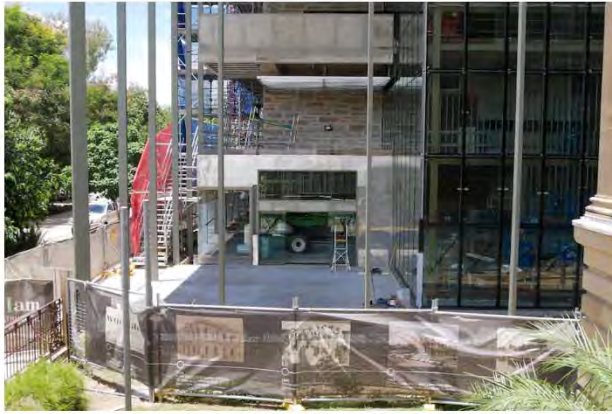
Construction of the new Rockhampton Museum of Art is expected to be completed by April. (ABC Capricornia: Rachel McGhee)
